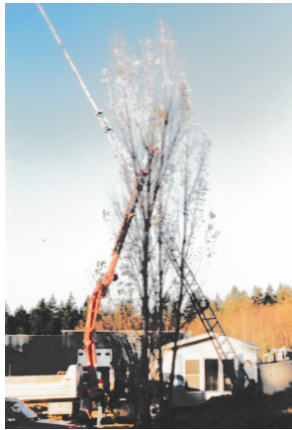
Up she goes with a scramble at the tower's base to bolt it down!
