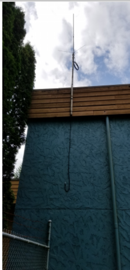
The antenna is on the South East side of the building.
