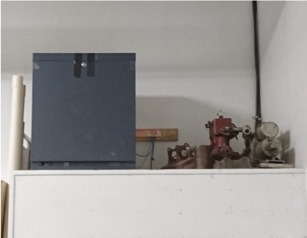
The repeater is bolted on top of the fire hall's communication cabinet.
