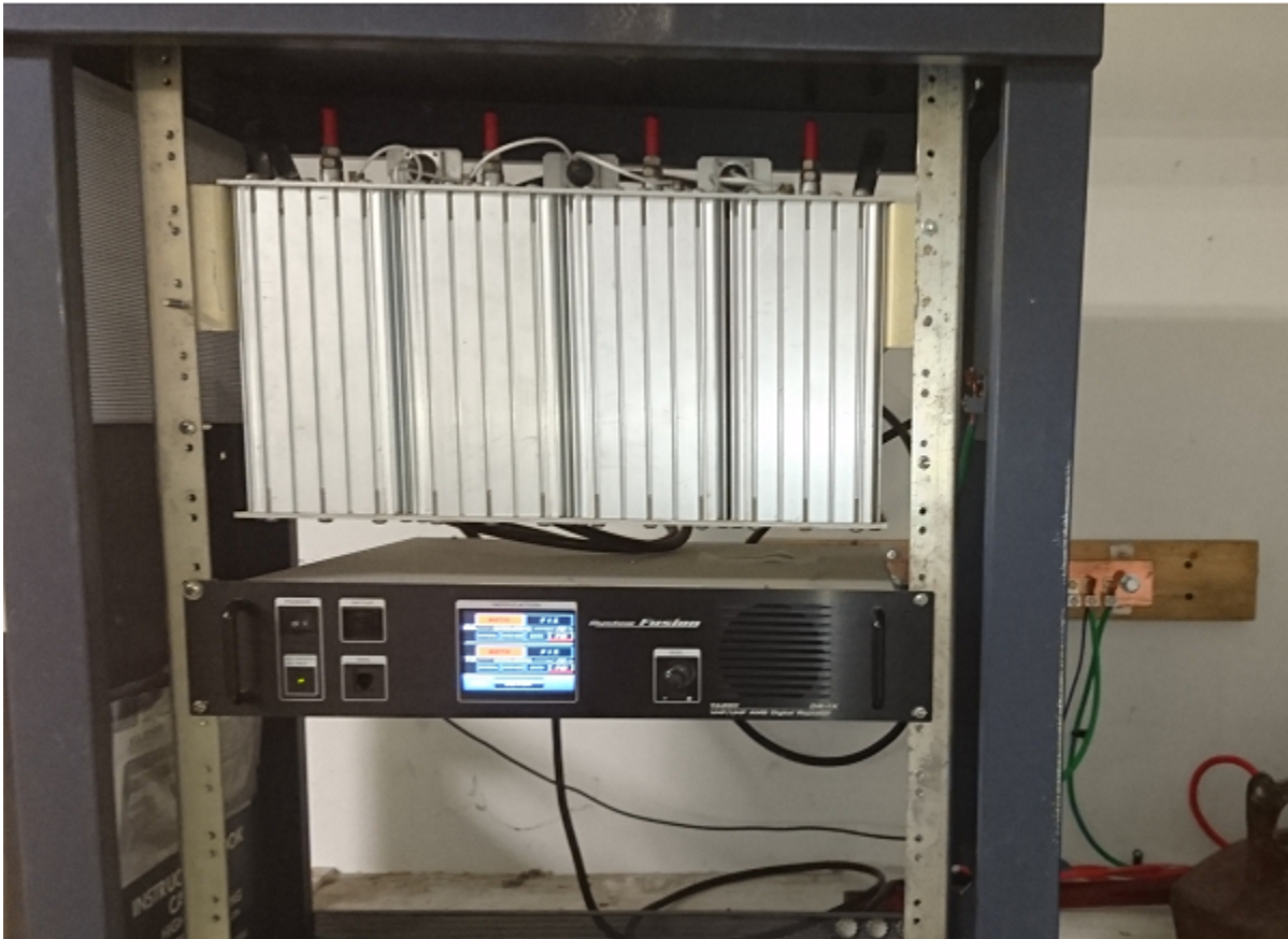
It is all self contained with power from the grid and a battery for backup (not shown here)
