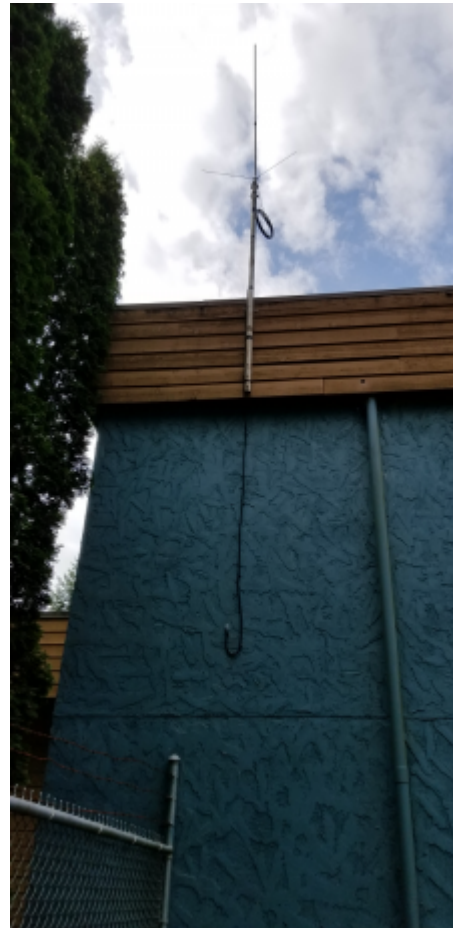
The antenna is on the South East side of the building.
