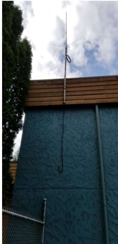
The antenna is on the South East side of the building. here )
