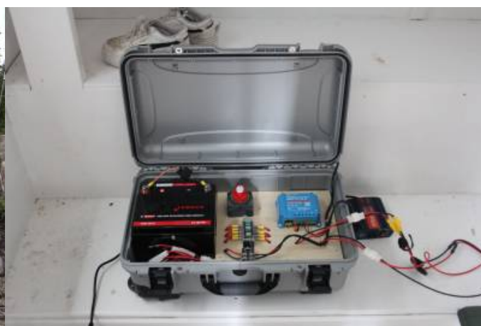
VE7LDB's solar battery box
